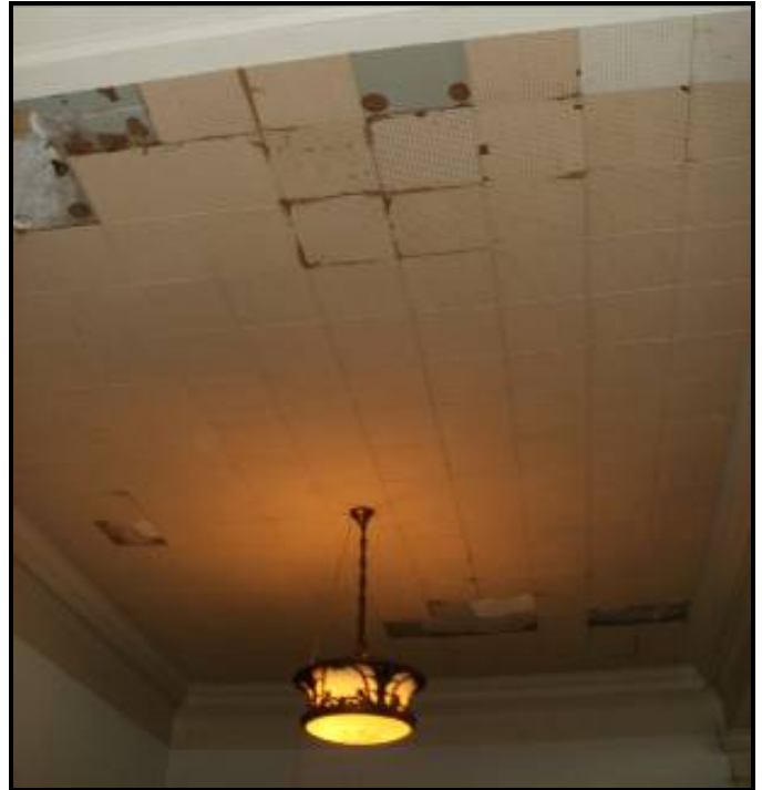
East Stairwell Ceiling – Needing Repair
